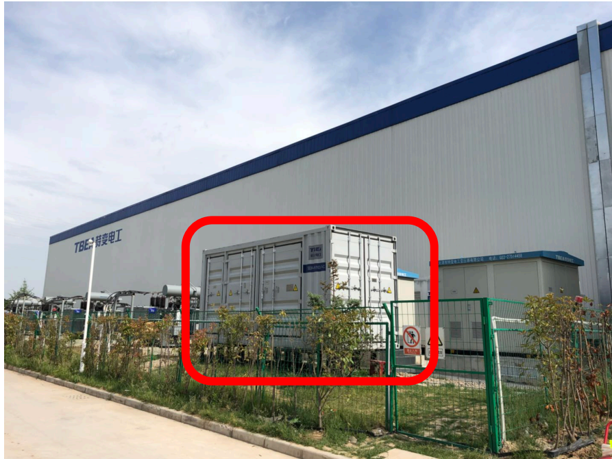
The PE transformer installed in TBEA Park
